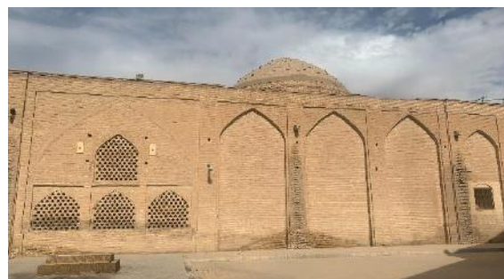
Fig. 20. Using materials with minimal risk of falling in the facade of the mosque
